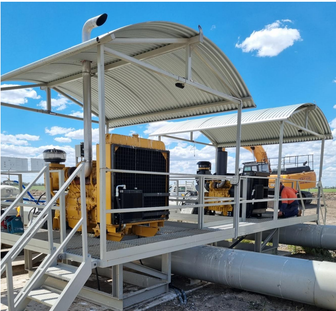
Figure 13 - Remote control and monitoring of diesel pumps by McGregor Diesel
